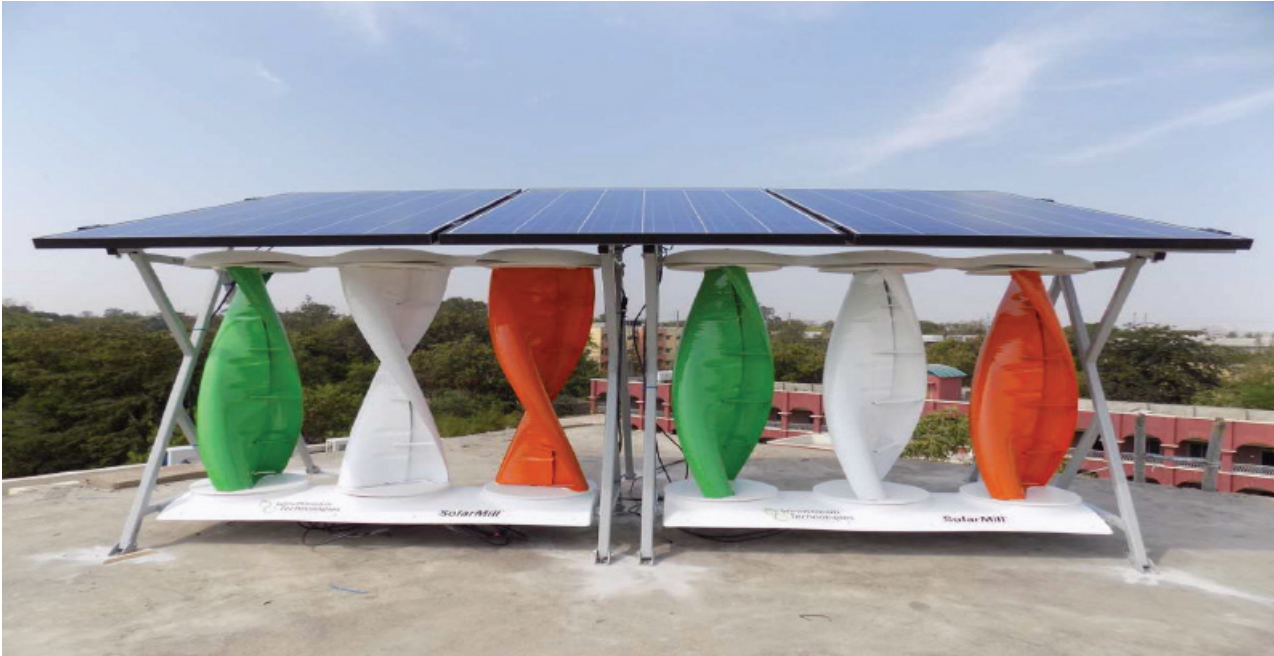
Figure 58: Solar wind hybrid system
