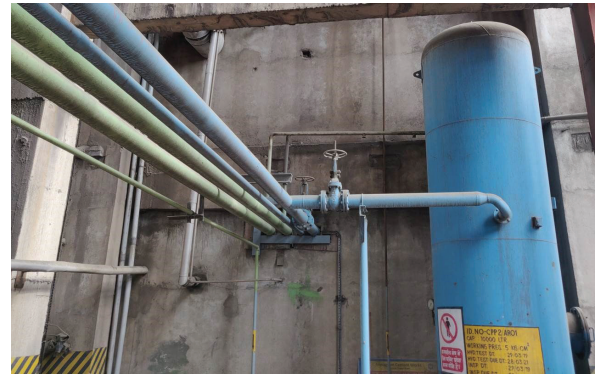
Figure 46: Existing compressed air piping
