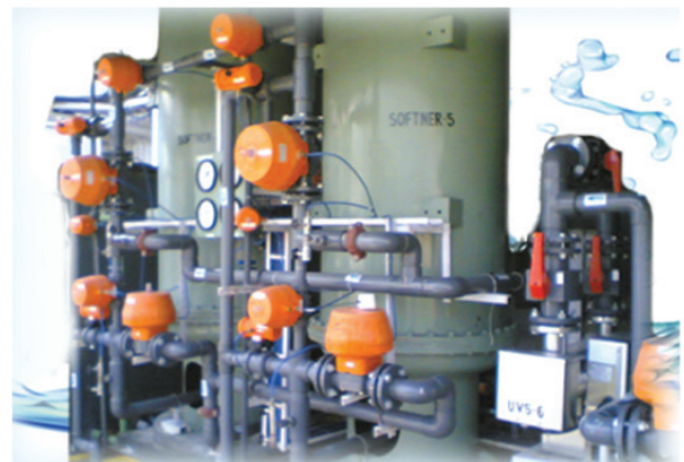
Figure 70: Water softener unit
