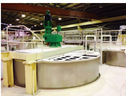
Figure 15: Slip agitation and storage
