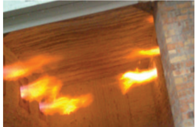
Figure 69: Improper air to fuel ratio
